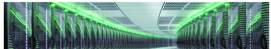
Data center cooling
